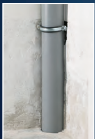
1. HT / KG pipe 33 cm cut out
